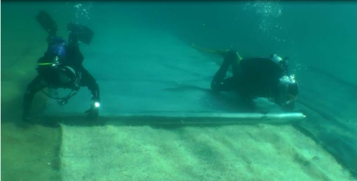
Figure 4. SCUBA diver installation of Curlex (light material in foreground) and EPDM benthic barrier (dark material behind divers) over the sill of Emerald Bay. Photo from Zabaglo 2015.
